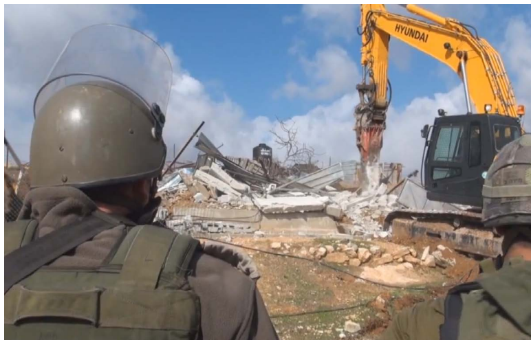
[illustration 4] Hyundai construction vehicle being used to demolish Palestinian houses in Beit Hanina, Occupied East Jerusalem on November 24, 2011.
